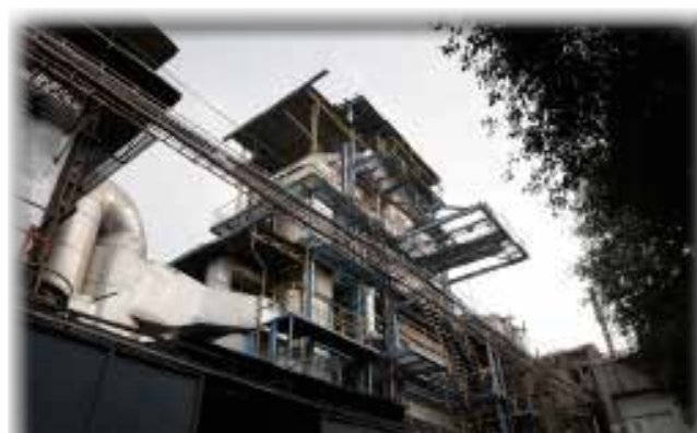
Co-Gen plant for Turbine Generator MIL unit-1 Hapur
