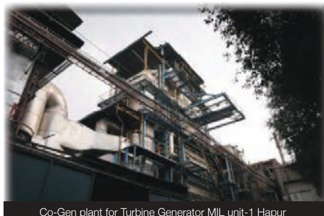
Co-Gen plant for Turbine Generator MIL unit-1 Hapur
