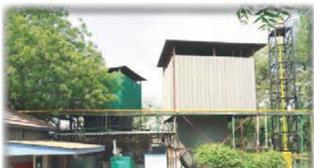
Bio Gas plant at MIL unit-1
