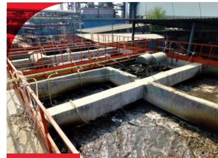
ETP to treat Industrial Waste Water- Merino Industries- Hapur
