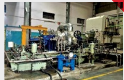
Biomass based Turbine, Hapur
