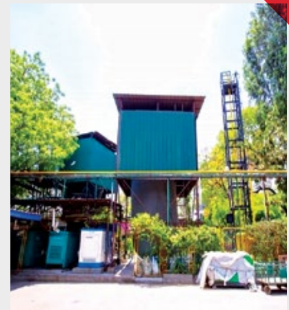
Biogas system, MIL Hapur
