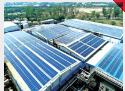
Rooftop Solar, MIL Hapur
